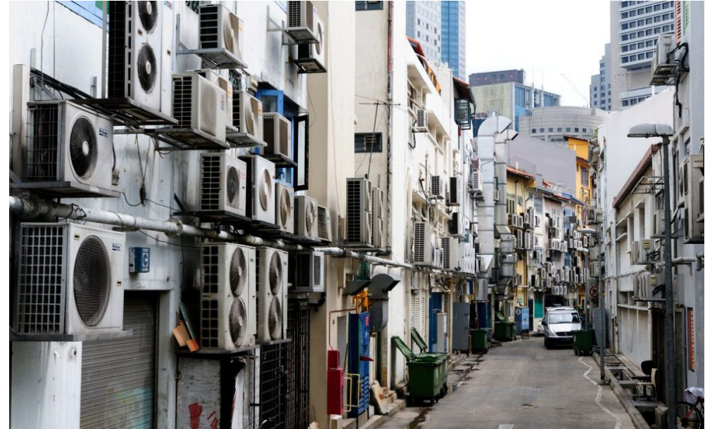
Air conditioning in Singapore
